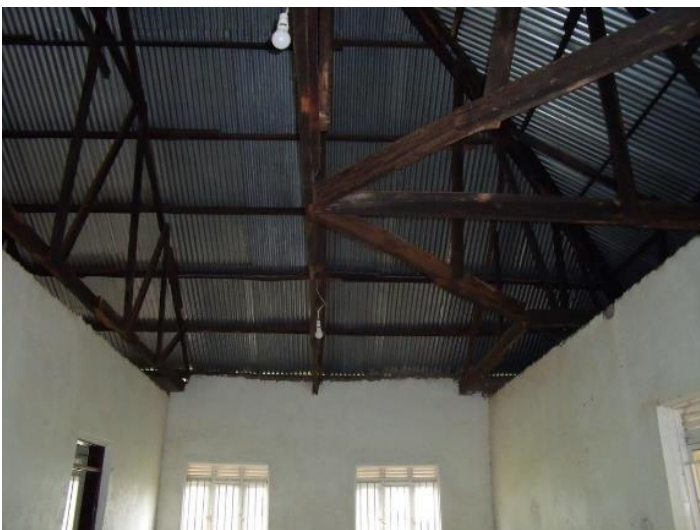
Inside of the hostel showing the lack of a ceiling
