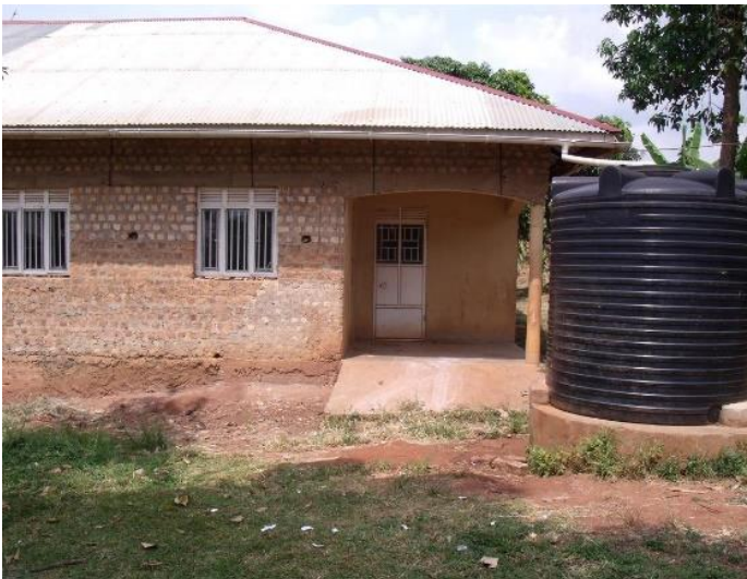
Water tank and girls' side entrance. This wall also needs plastering and an apron
