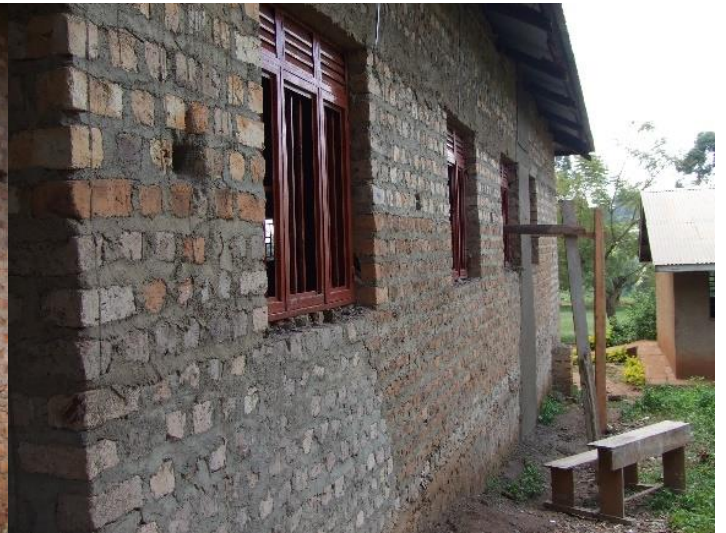
One side wall of the hostel which requires plastering and an apron at base of wall
